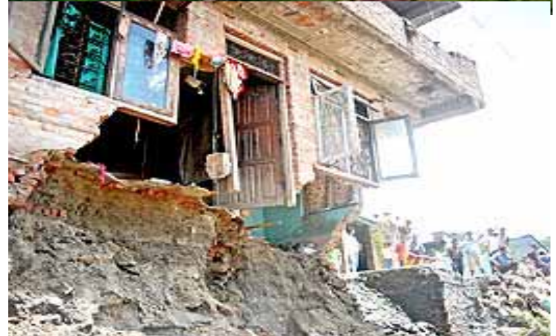
Damage caused by landslide
